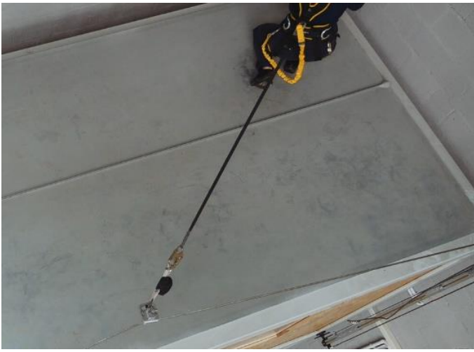
Work restraint on container roofs
